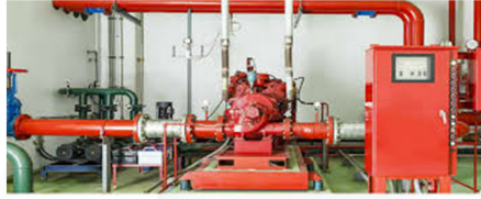
Fire Hydrant System
